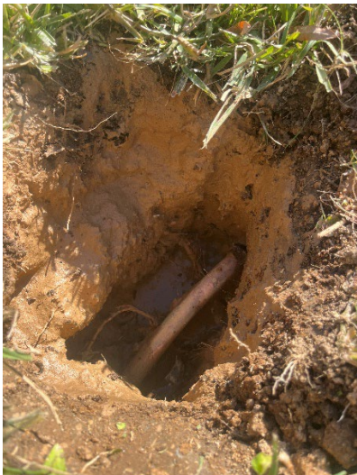
Copper Service Line Material
